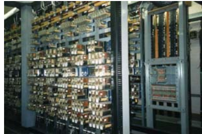
Relay interlocking Constructed with complex circuitry made up of relays
